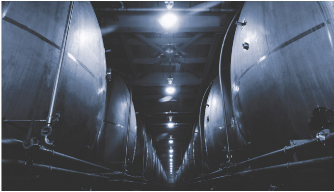
Fill level measurement in tanks
